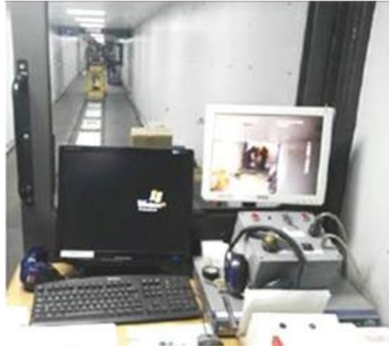
Figure: 23. Fire Control System
